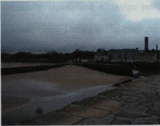
Plate 6.7: Sediment Piled Between Cross Pier and Breakwater
