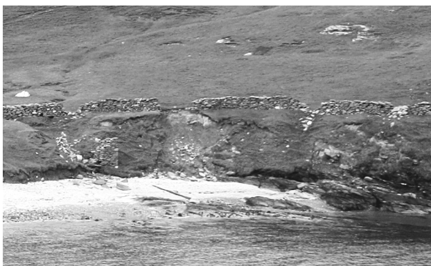
Figure 5. Same view as Figure 4, taken in 2010. Much of the building has collapsed due to erosion below one corner (copyright Tom Dawson).
