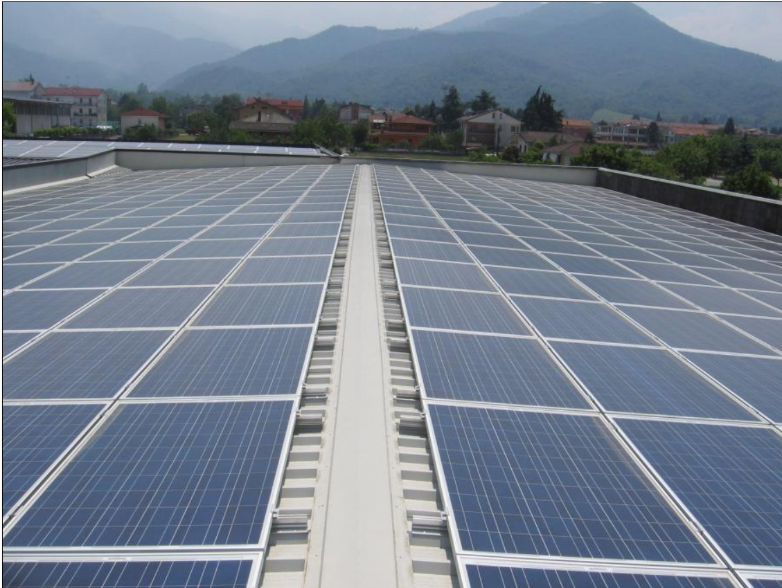
Figure 9. Rooftop solar plant in Boves, Piedmont.
