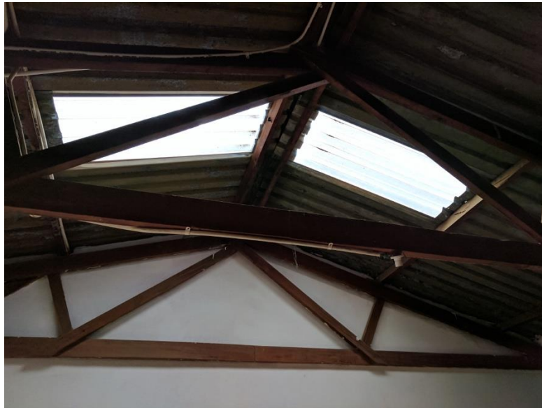
Figure 4: Transparent roofing tiles in a classroom.
