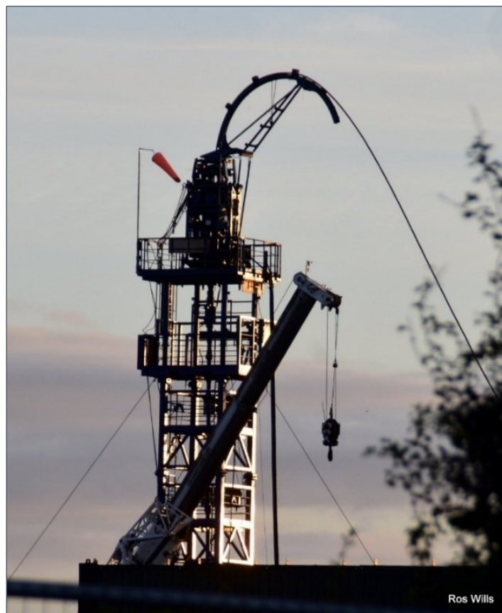
Figure 2: Close-up of the workover rig, from the roadside, September 2019. Credit: Ros Wills
