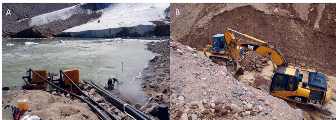
Fig. 13. Preventive work on the MGL in the Ile Alatau: A - the MGL N°13-bis (U. Almaty River basin) water pumping by and siphons, B – deepening of the evacuation channel for emptying the MGL N°6 (the K. Almaty River basin); source: Medeu et al. (2018).
