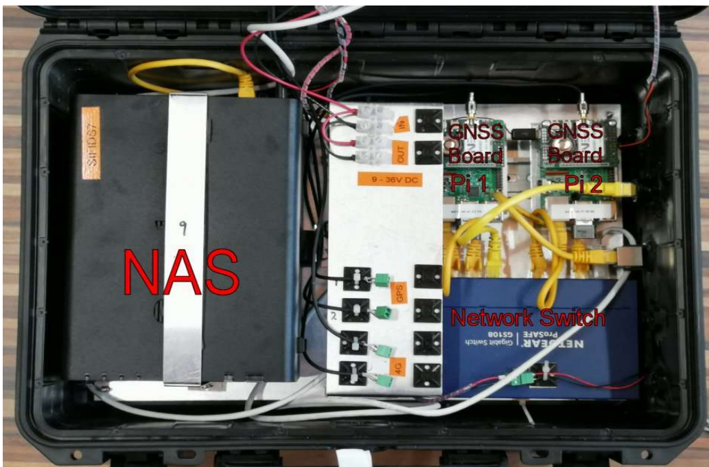
Figure 7. Base of completed logger unit, note the incoming power and antennae leads were removed for clarity.
