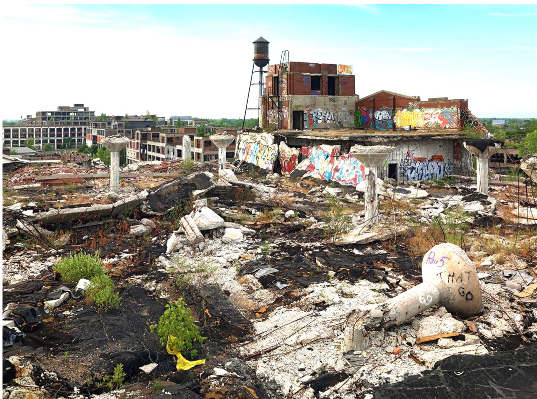
Figure 4 Packard Automotive Plant, Detroit, Michigan. Dave Jordano, Collapsed Roof, Packard Automotive Plant, Eastside, Detroit 2012 , photograph, Dave Jordano (blog), accessed 29 August 2018, https://davejordano.com/detroit-unbroken-down/detroit-unbroken-down-4-2012- .
