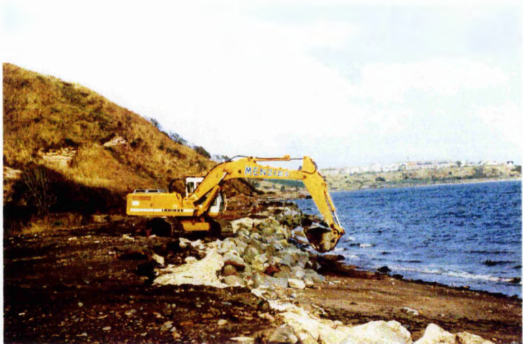
Plate 2.23 Remedial work was carried out by Fife Council to protect the live sewer and track road to the gasworks in 1993. Erosion of the material behind the riprap is visible in the lighter coloured areas on the left of the picture, where the sediment has been washed away. This picture highlights how some of the actions carried out by Fife Council encouraged further instability of the coastline as opposed to stabilising it.
