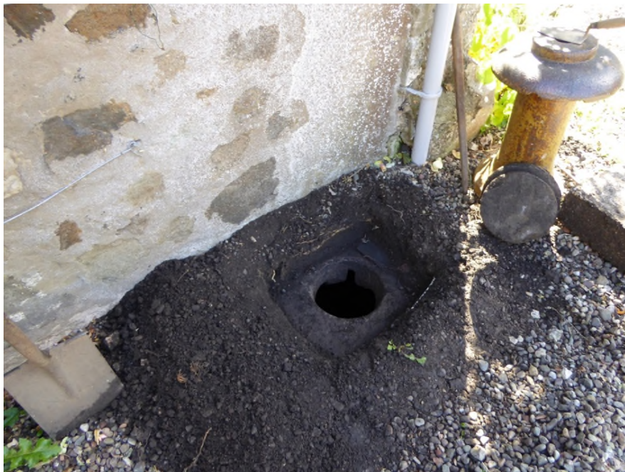
Ph. 1.10.1 © PR The well at the house wall, uncovered.
