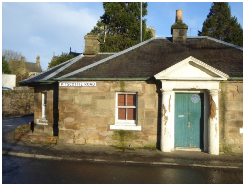
Ph. 2.17 © PR East Toll-house, Cupar: one original gate-post is visible in the far wall on the LHS of the toll-house. The plaque inscription reads: Built c. 1825 to collect tolls from travellers on the turnpike roads to St Andrews and Pitscottie. Tolls were charged here from 1791 until they were abolished in 1878.
