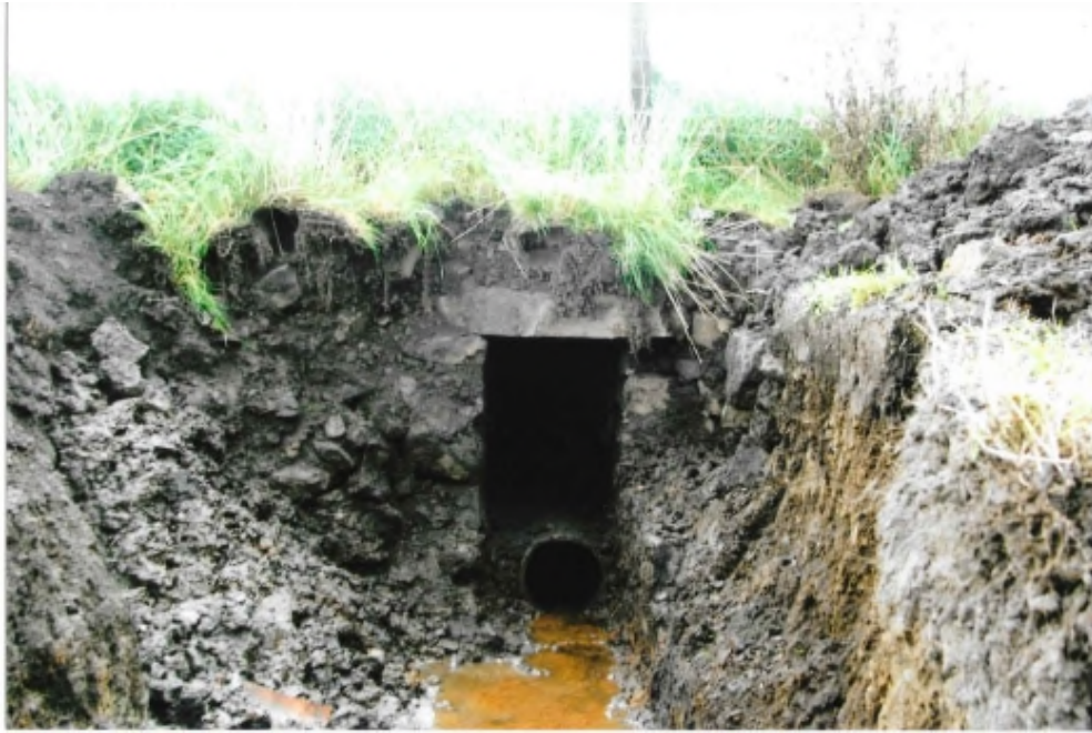
Ph. 1.20 © T&MG The big drain under the south drive, draining the former moss area.
